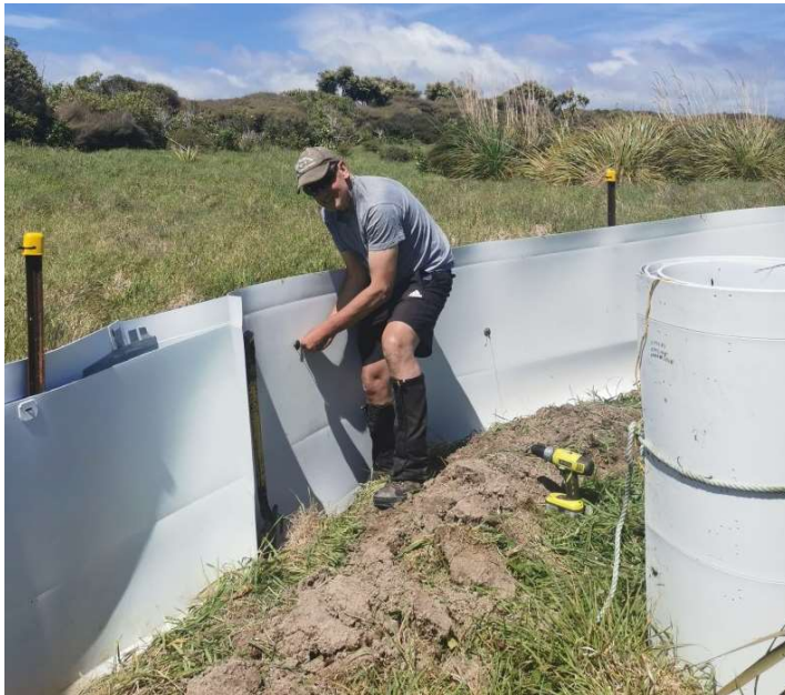
Colin Miskelly attaching new (recycled) cladding to the inside of weevil MIQ fence, October 2022. Image: Annemieke Hendriks
